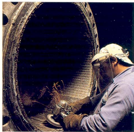
Blast furnace piping
